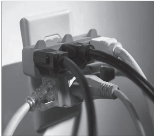
Don't overload your electrical system and outlets.
